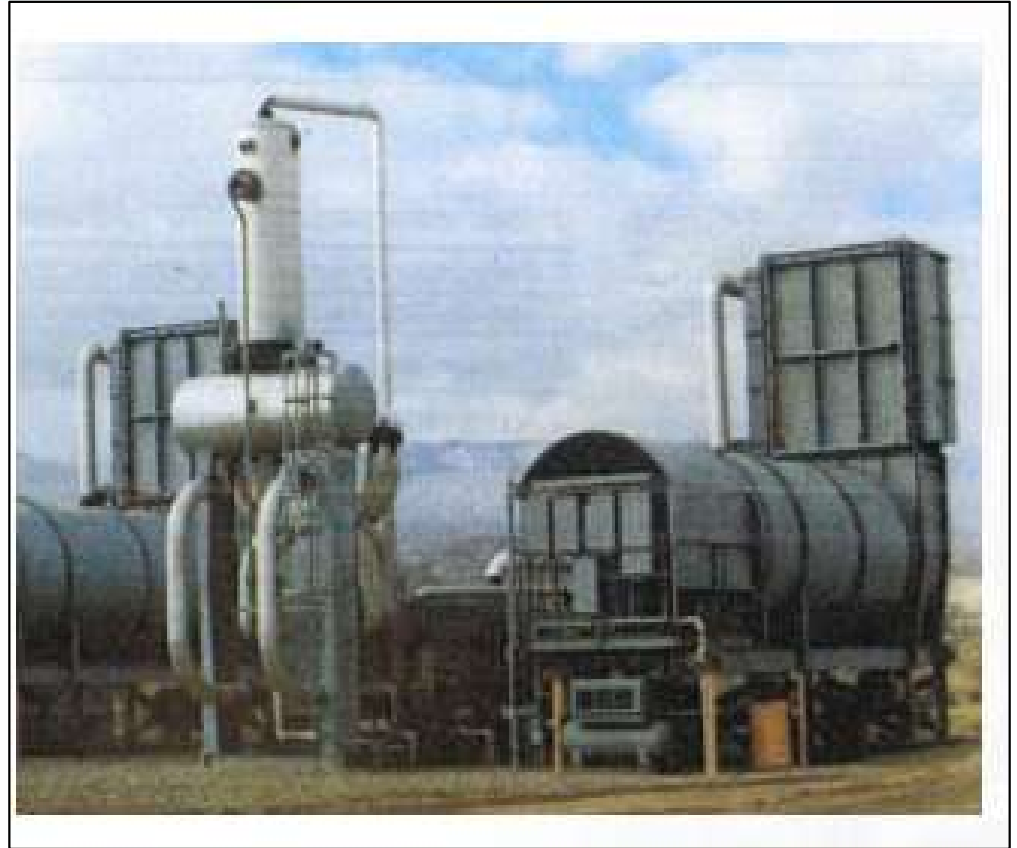
“Thermosludge” Boiler – California 1970's
